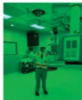
Green lighting in the hospital's operating room reduces the intense brightness, resulting in less fatigue for doctors.
